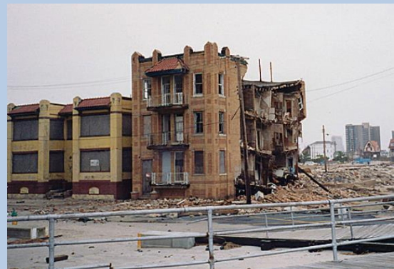
Boardwalk at Oriental Avenue, Atlantic City, days after the December 1992 Nor'easter (Photo courtesy of Flickr user Pentax Travels).
